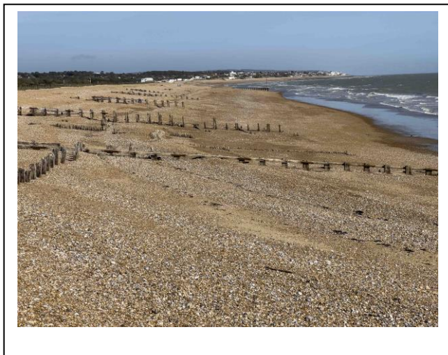
The sorry state of the groynes at Waller's Haven, Bexhill-on-Sea.
